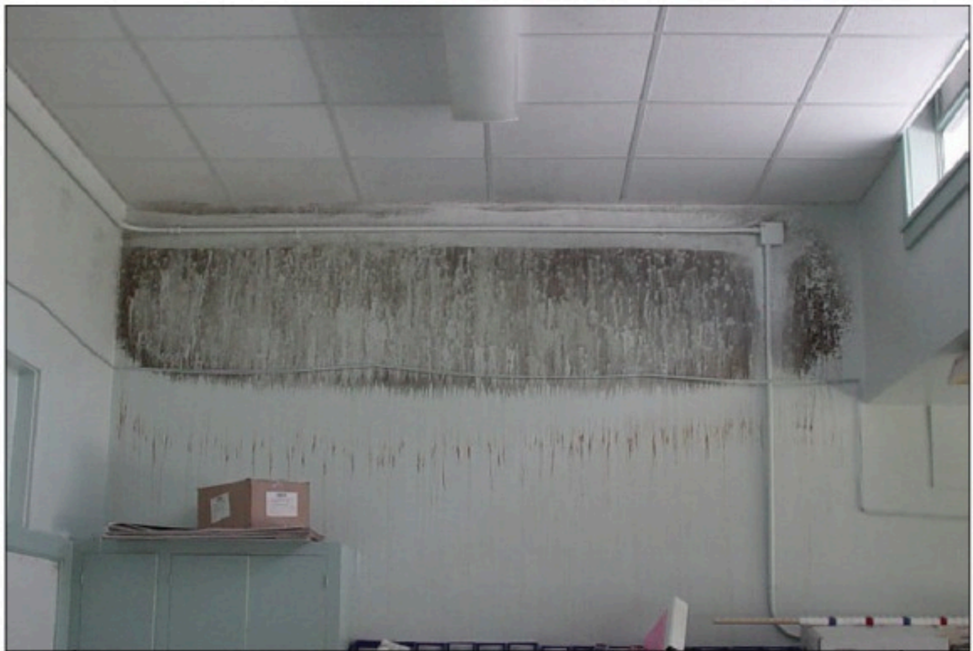
Photograph 1: Mold growth on classroom wall after 72 hours.
