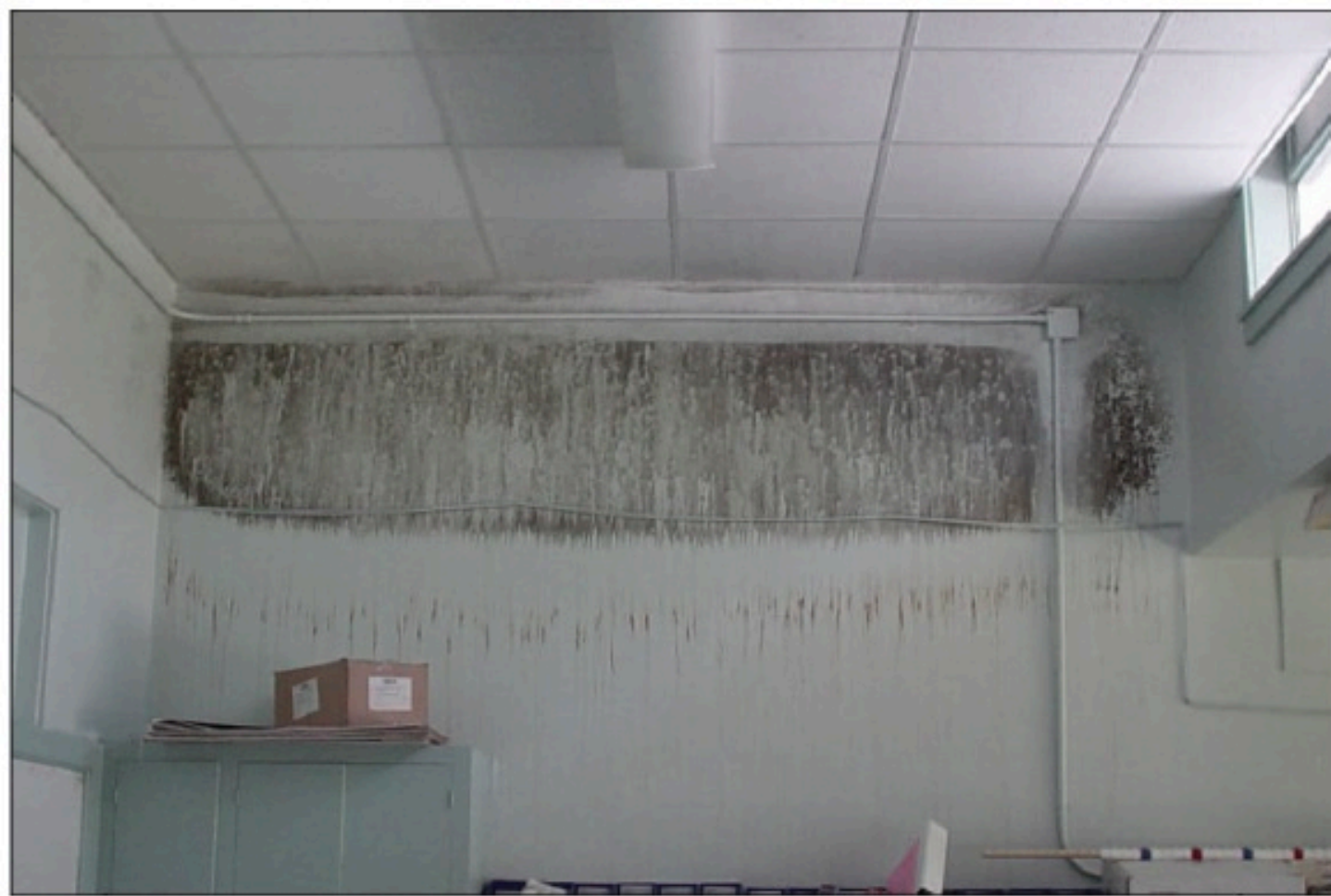
Photograph 1: Mold growth on classroom wall after 72 hours.
