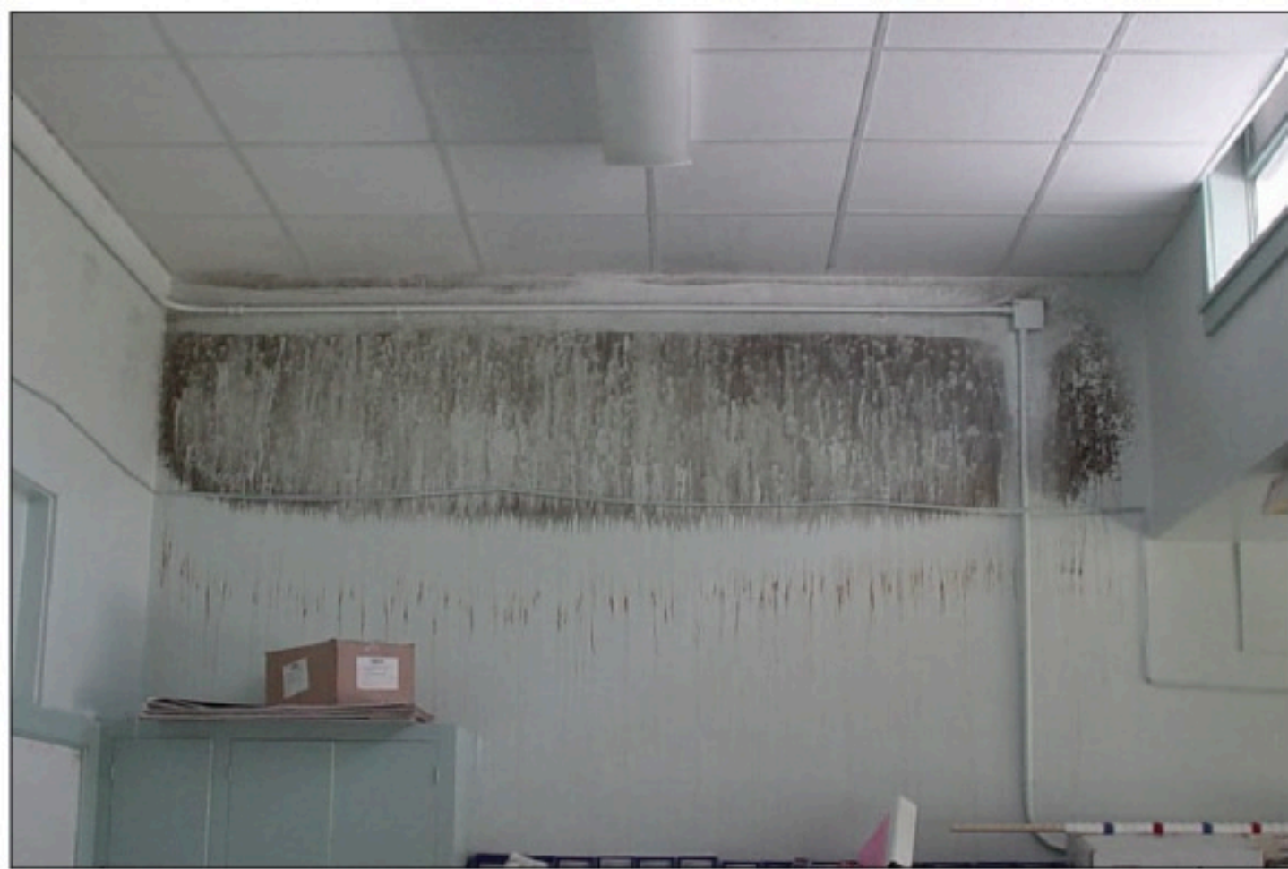
Photograph 1: Mold growth on classroom wall after 72 hours.
